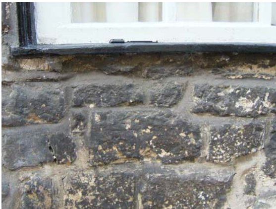
Thick black crusts on Headington freestone in a sheltered portion of wall under a window sill of a south-facing cottage on Hollywell Street.
