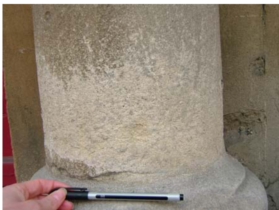
Pitting, roughened texture at base of column – possibly caused by salt weathering, Beaumont Street.
