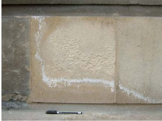
Salt tide and roughened flaking surface caused by salt weathering, Beaumont Street.
