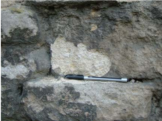
Blistering of stone encrusted with black, gypsum-rich crust, St. John's College.
