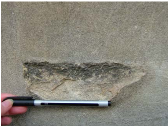
A blister/scaling developed on ashlar block, Beaumont Street.
