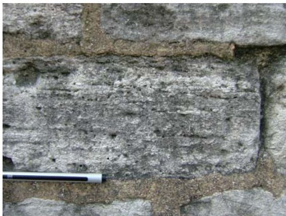
Pitting orientated along bedding planes, St. John's College.
