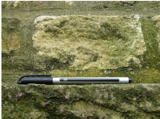
Green algal cover on stone and mortar, St. John's College.
