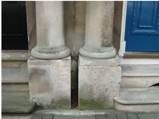
Left hand column base shows roughening due to salt weathering on right hand side, Beaumont Street.
