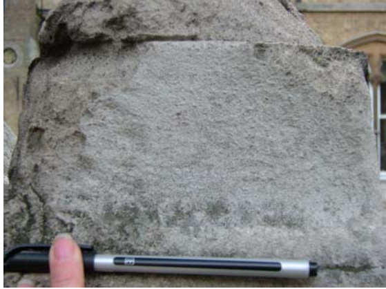
Erosion of corners of balustrade – after intense gypsum crust development and cleaning, Ashmolean Museum.
