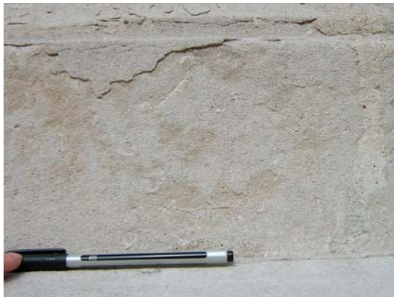
Flaking of Bath stone after cleaning, Ashmolean Museum.
