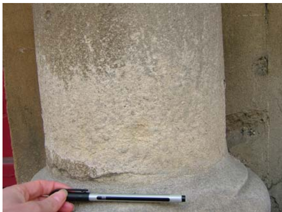
Pitting, roughened texture at base of column – possibly caused by salt weathering, Beaumont Street.
