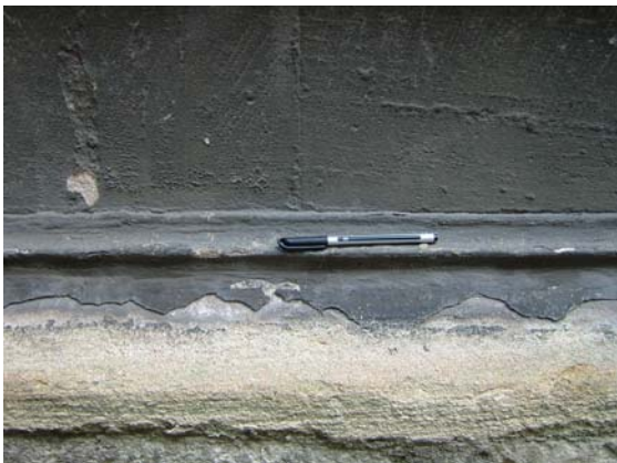
Black encrustation intact, in a sheltered section of a west-facing wall at the University Church of St. Mary the Virgin, but peeling and removed where the plinth protrudes.
