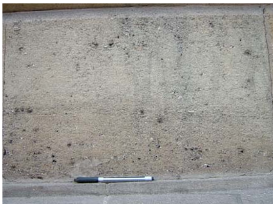
Blackened pits visible on the north-facing façade of Oriel College on High Street.
