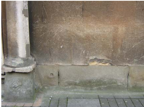
Serious erosion of sandstone plinth underlying limestone ashlar and columns, Beaumont Street.
