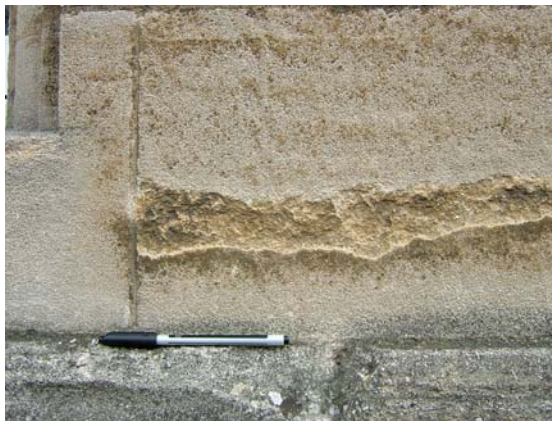
Flaking of ashlar block, St. John's College.
