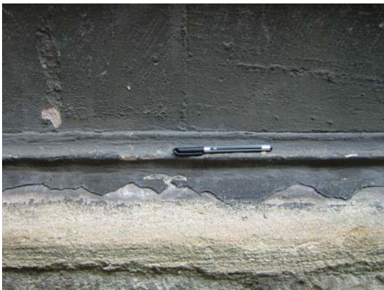
Black encrustation intact, in a sheltered section of a west-facing wall at the University Church of St. Mary the Virgin, but peeling and removed where the plinth protrudes.
