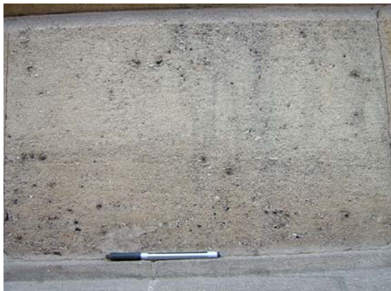
Blackened pits visible on the north-facing façade of Oriel College on High Street.
