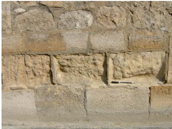
Cavernous weathering in the boundary wall of Magdalen College on the east side of Longwall Street, with mortar standing proud of friable and crumbling blocks of recently cleaned limestone.
