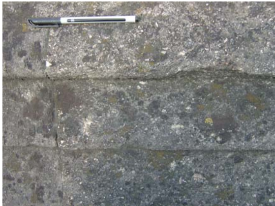
Close-up of the variety of lichens growing lower down on the string course.
