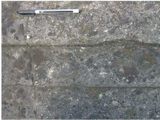
Close-up of the variety of lichens growing lower down on the string course.
