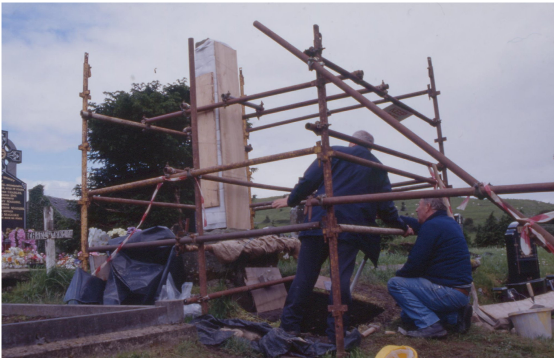
Plate Seven: Engineering work to correct the High Cross's tilt in progress.
