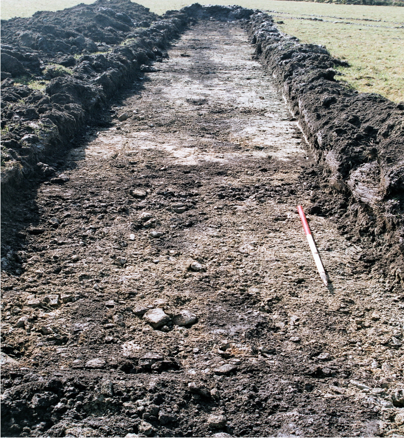
Plate 3: View of Trench B from north, after excavation to surface of subsoil (C202). The faint trace of two plough furrows can be seen running north-south along the trench.
