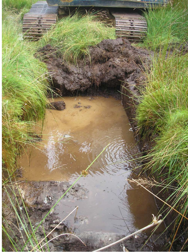
Plate Five: Trench One following excavation to subsoil (Context No. 103), looking north-east
