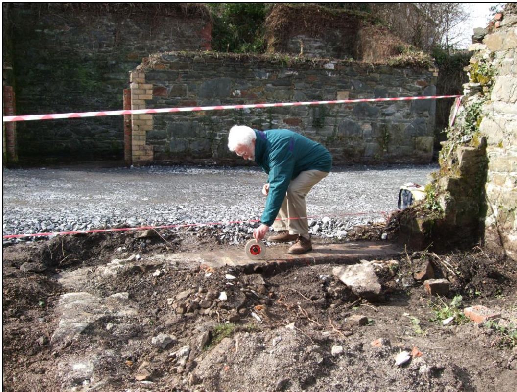
Fig. 15: Purifier house looking east (March 2011): the tape box rests on the threshold directly above the exiting pipe. (DSCF054).
