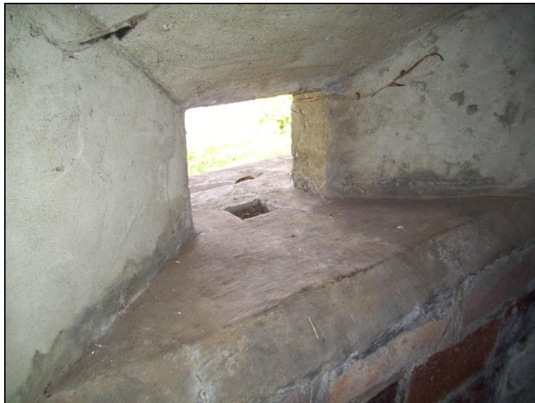
Figure 15: Inside a Type 22 Pillbox in Elstead, Surrey, complete with concrete loopole tables (Pillbox Study Group)
