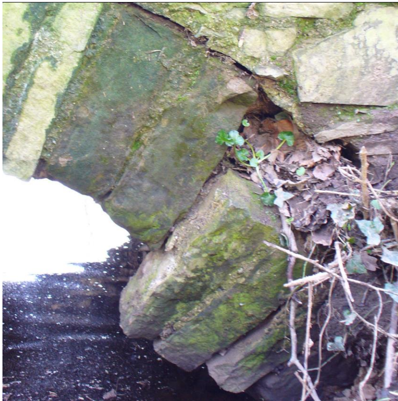
Figure 13: Damage to north-eastern face abutment
