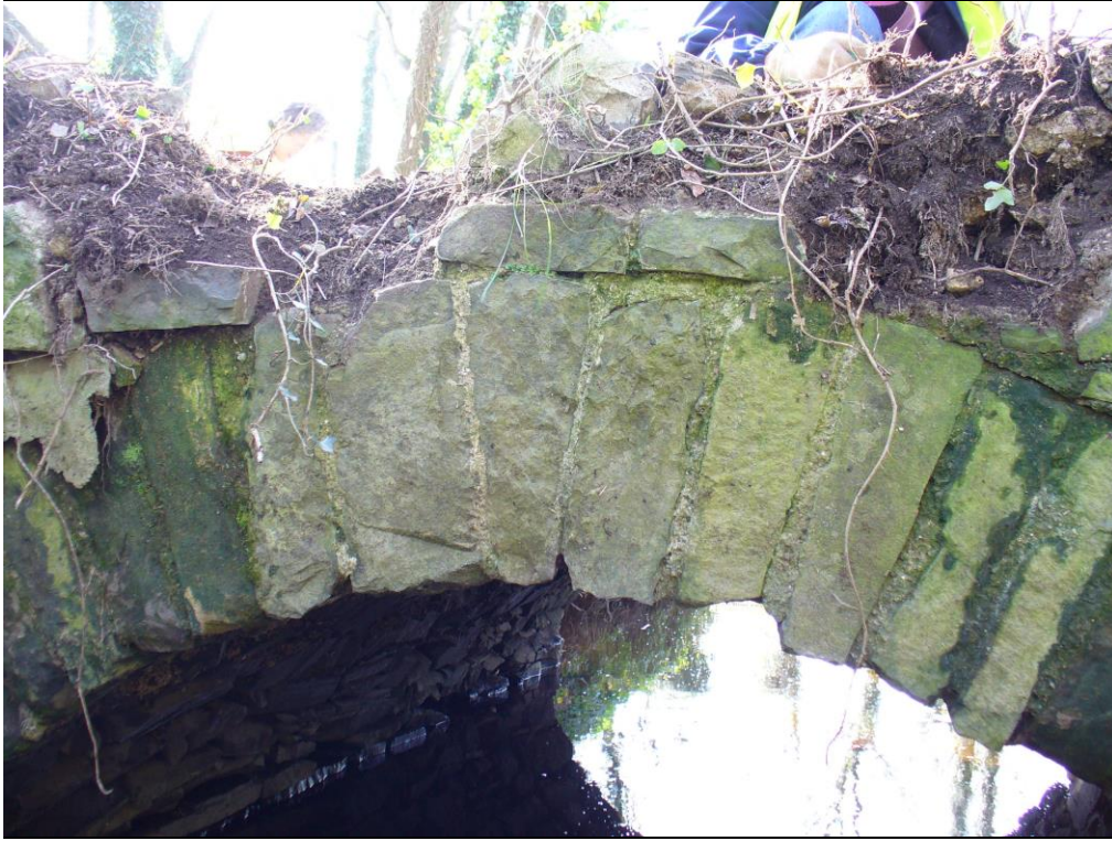
Figure 14: Damage to parapet on north-eastern face
