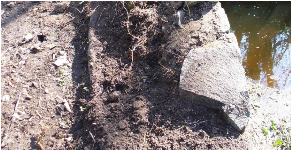
Figure 09: Example of root damage to bridge deck.
