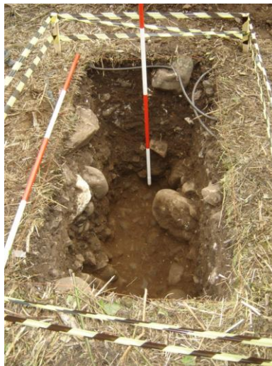
Low-level hazard tape presenting a trip hazard
